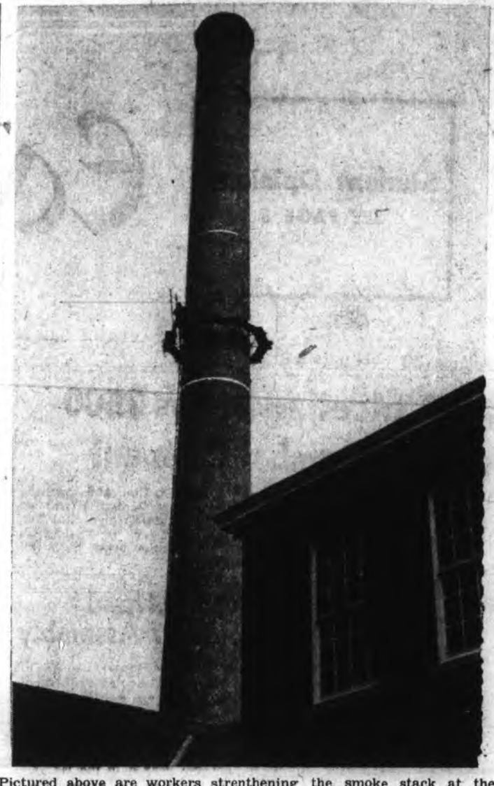
Pictured above are workers strengthening the smoke stack at the heating plant. Once this work has been completed, the college will be able to double the heating capacity of the college.
