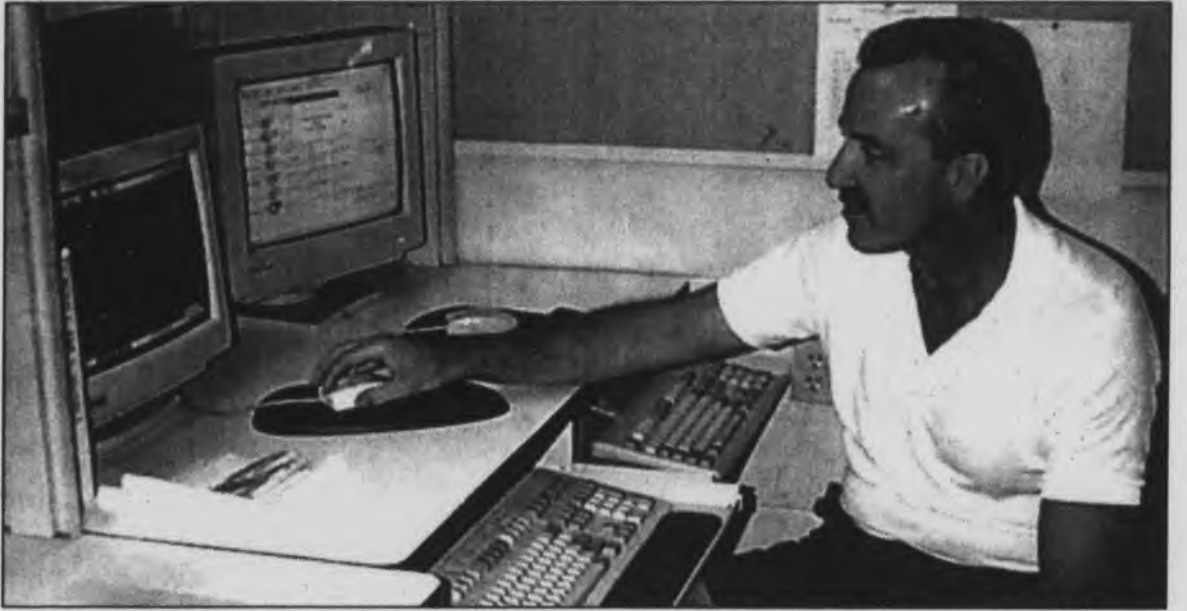
Steve Allen spent his labor day watching computers that monitor campus. Allen is operations coordinator for Eastern's physical plant. He said that the computers, which monitor environmental conditions on campus, are watched at all times in case of an emergency. If a life-threatening or property damage situation were to occur, Allen could dispatch maintenance personnel. Allen said that if he were not working he would like to spend Labor Day with his wife and family.
