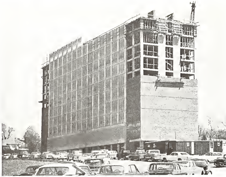
This 13-story girl's dormitory is expected to be ready for the fall semester. It is the first of four in an $11.5 million complex designed for 2,400 women. A similar plan is underway for a men's complex. The girl's dorm will be named the Brown Tellord Dormitory, honoring a former Eastern faculty member.
