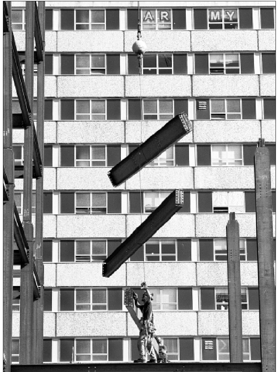
GOING UP – Chan Isaacs with Wylie Steel of Nashville, Tenn., guides steel supports as construction continues on the new Student Services Building. The building, expected to be completed by Spring 2002, will house a variety of offices that serve students and will include a 400-seat multi-purpose auditorium.
