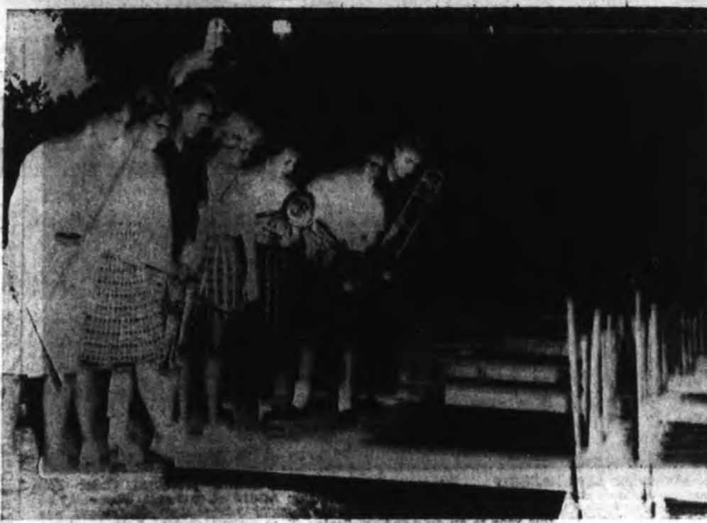
IT WON'T BE LONG NOW... Members of the Eastern Kentucky State College Band watch as the foundation is being poured for the James E. Van Puersem Band Pavilion. Named in honor of the head of the music department, the pavilion is expected to be completed in December.
