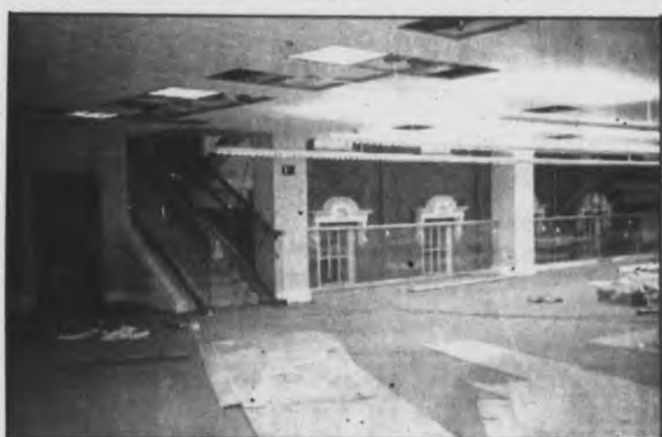
Photo submitted SNEAK PREVIEW—No tours of the library's new section are currently being offered, but staff have been permitted to check out their areas. Construction is still under way on the expansion, and no date has been set for an opening.
