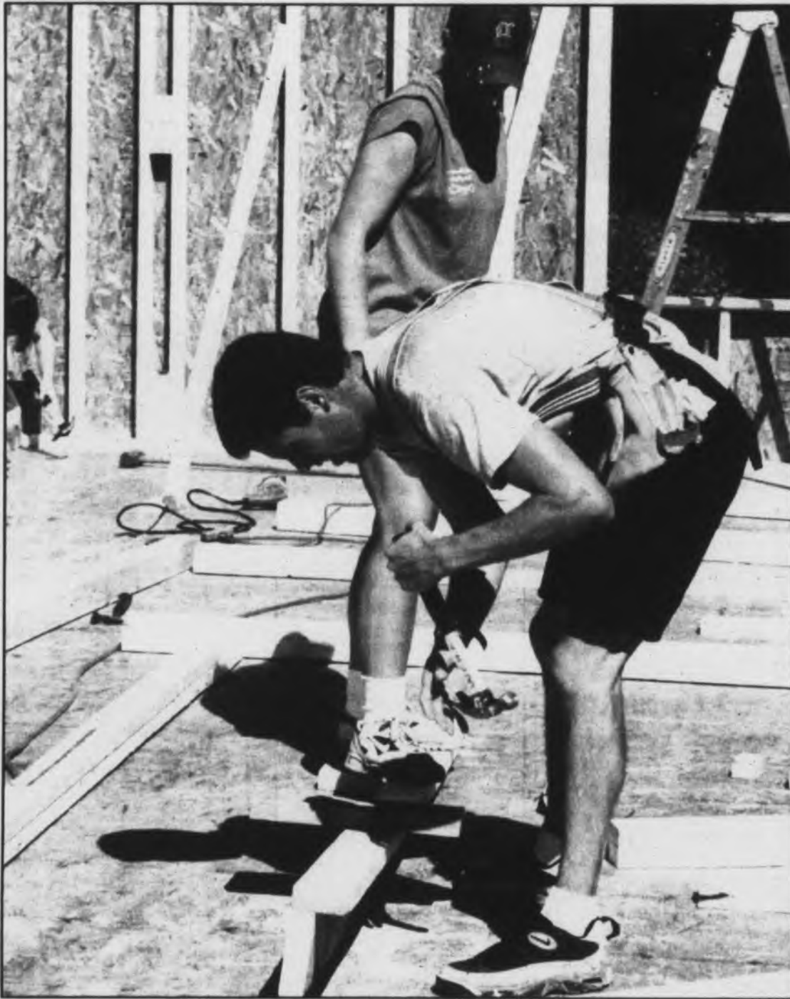
Habitat for Humanity volunteers work hard with community members to build houses for those who are in need.
