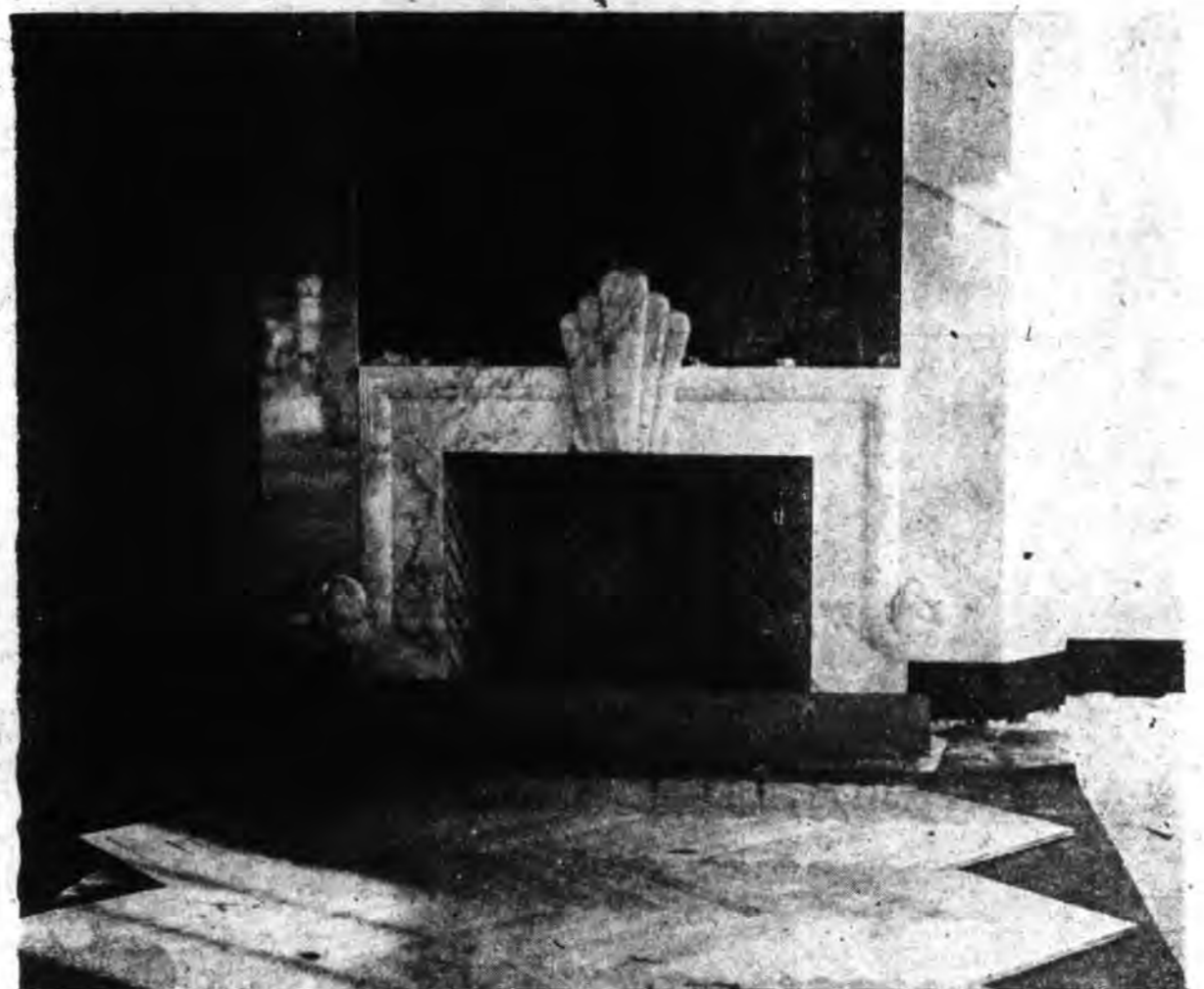
One of the doors in the banquet hall is shown in top photo with Harry Talamini, in charge of the marble work installation, and one of the workmen standing nearby. Lower photo shows one of the fire places in the student lounge.
