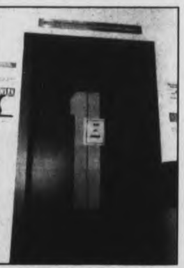
One of Commonwealth Hall's broken elevators
