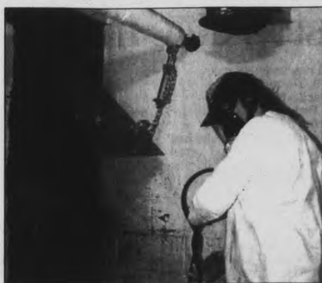
Coy Wells, a worker for Bio-Tech, prepares water and chemicals before cleaning the garbage chute in Dupree Hall.
