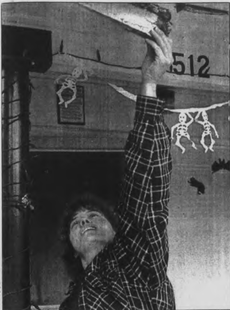
The roof of Deborah Glovak's Brockton home has several problems, some allowing animals to nest in it.
