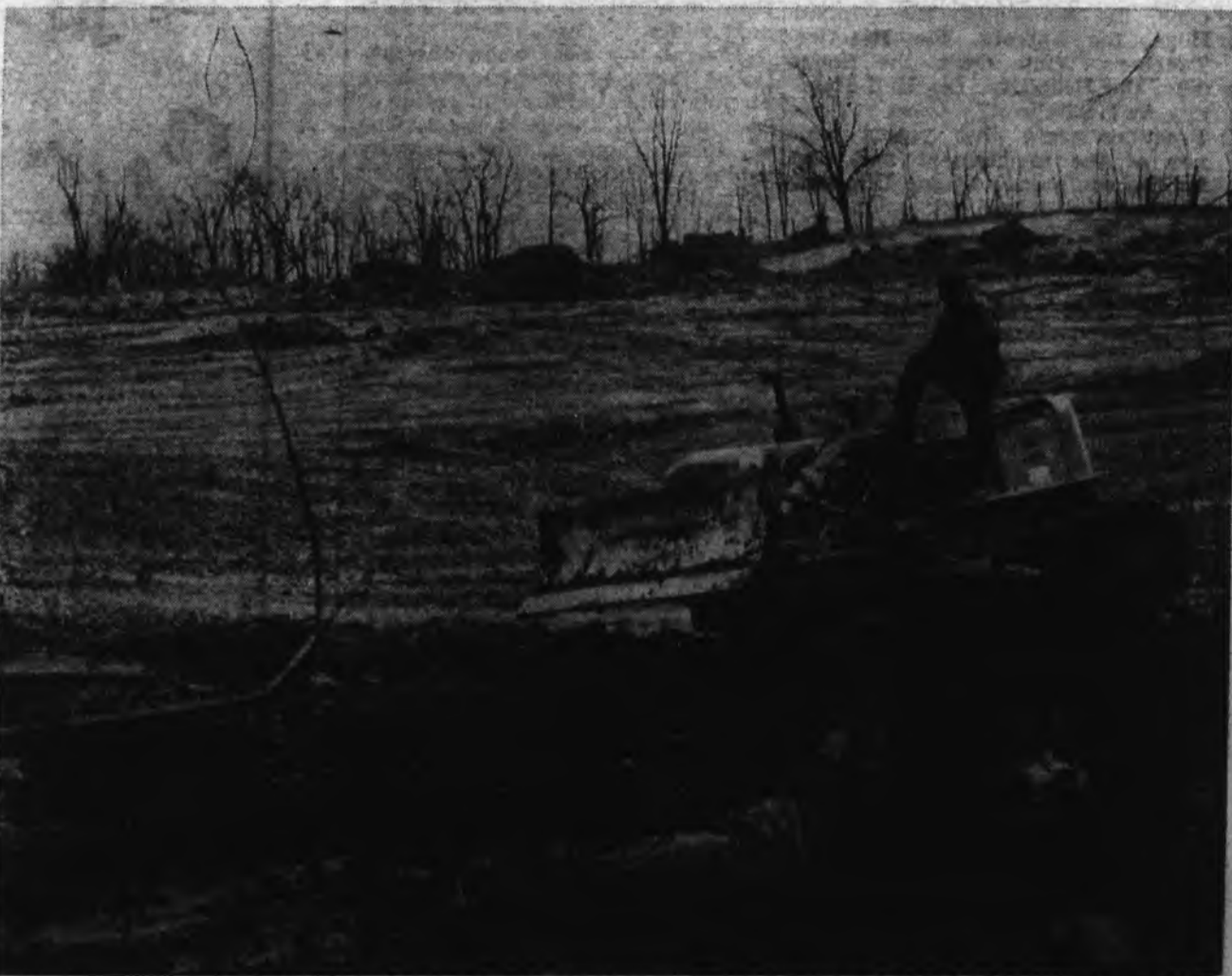
Excavation gets underway for the much anticipated housing facilities for married students.
