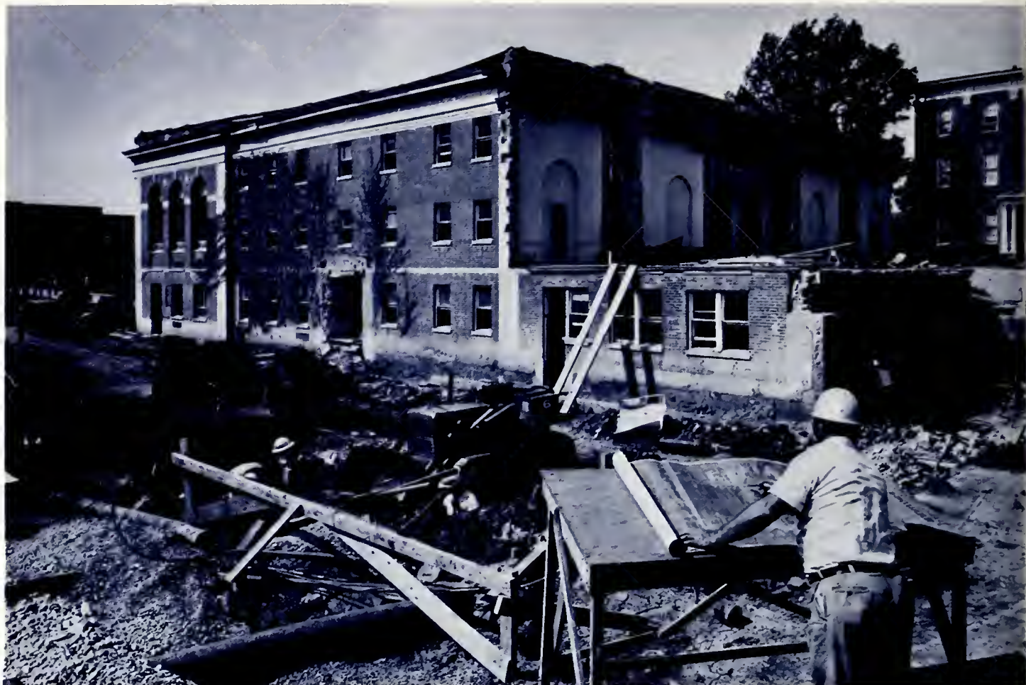
Campus construction continued with the reconstruction of the Crabbe Library, increasing its capacity to 500,000 volumes.
