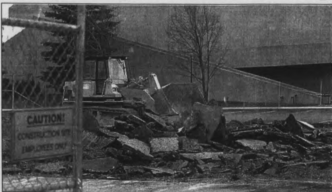
Dozers have been preparing the Begley parking lot for the new wellness building over the past week. The new structure is expected to be completed by June 13, 1999.
