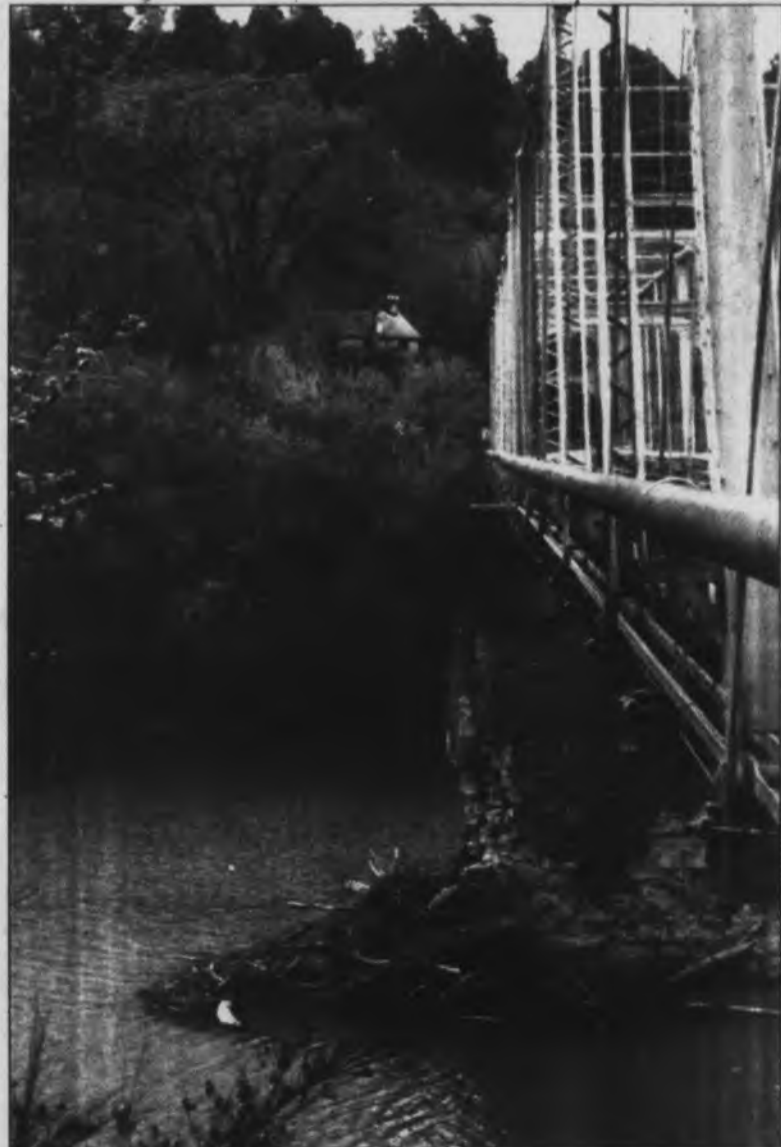
The foundation of the old Clays Ferry Bridge (above) is starting to fall apart, while trash floats down the river at Fort Boonesborough (above right).
