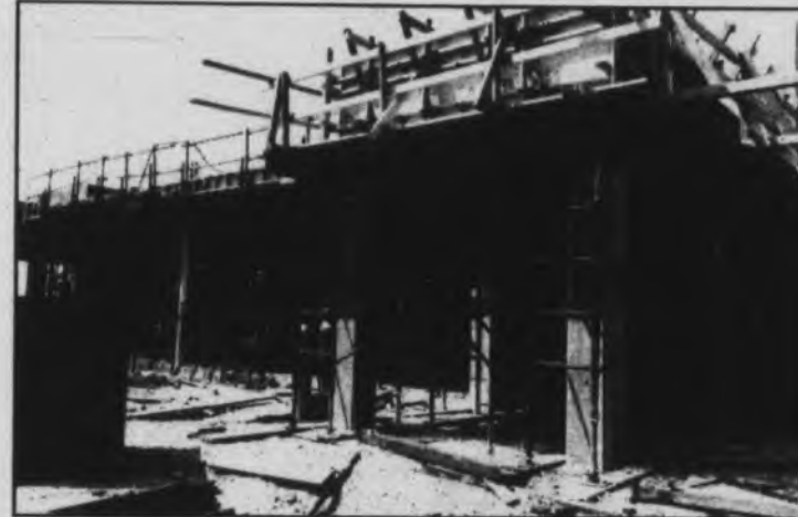
The university broke ground on April 13, 1990, to build a new nursing building. The $5.4 million building was needed to house the growing number of students in the allied health and nursing major.
