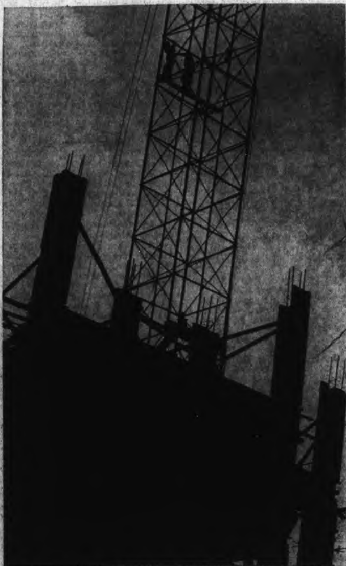
THE TOWERS CLIMB . . . Construction "zooms" on the new 12-story men's dorms, Todd and Dupree Halls, behind Alumni Coliseum. The twin dormitories, costing $2.9 million, will house 312 students each, and will be the tallest in the state. Both will be completely air-conditioned.
