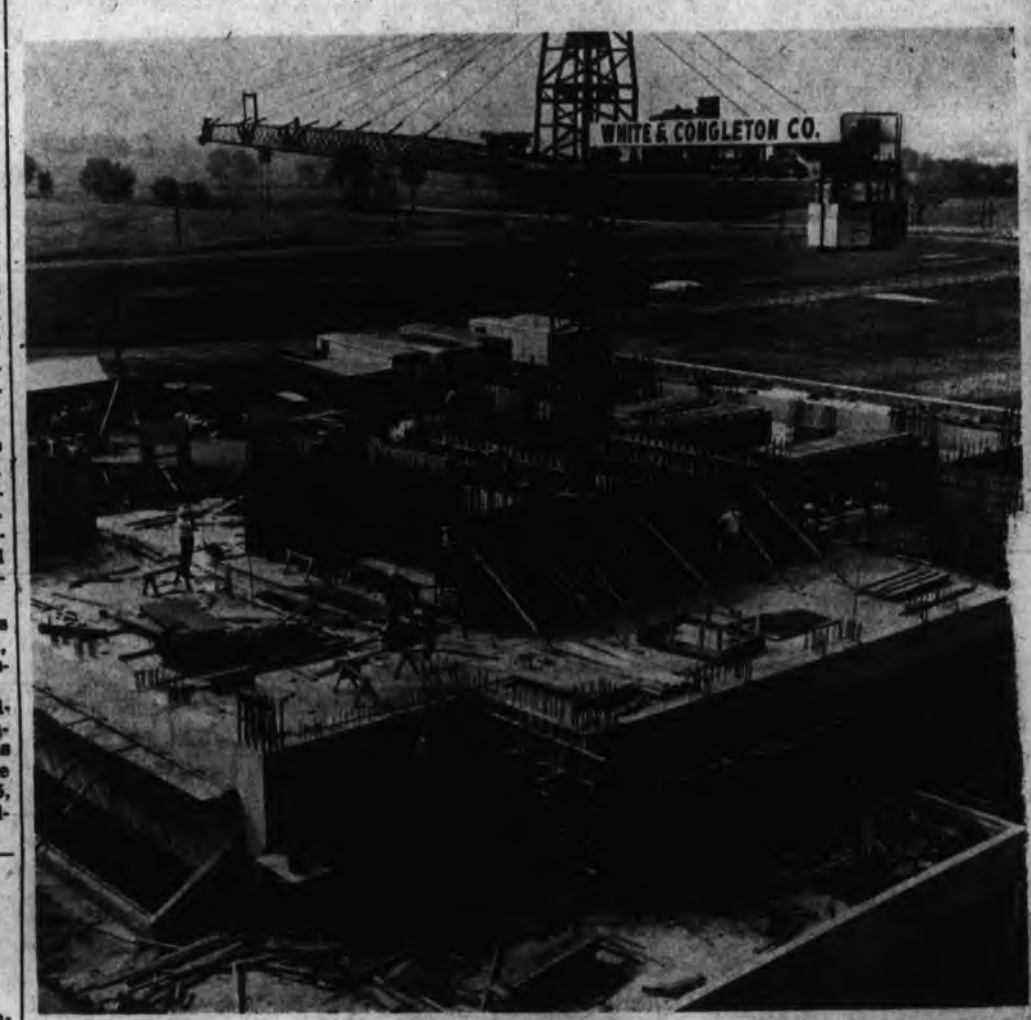
First Of Four This is the first of four dormitories to be constructed in the women's dormitory complex which will be completed about 1970. The complex will house 2,400 women, 600 in each of its four dorms. Construction will be underway sometime next year on the first hall in the complex.
