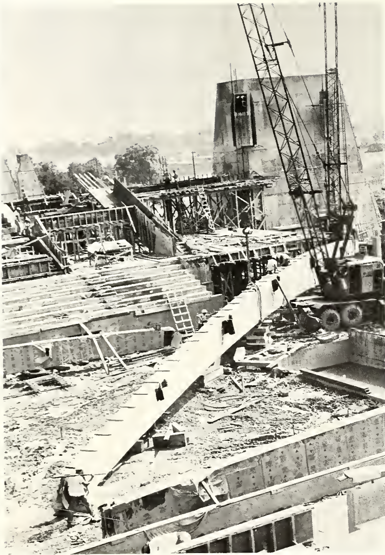
Disaster marked the construction of Alumni Coliseum; however, recuperation was successful.
