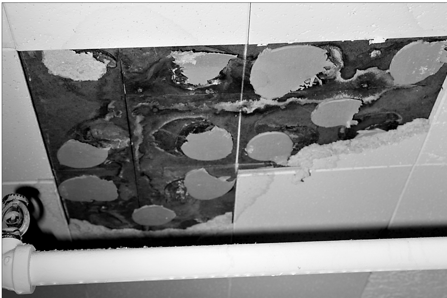
Ceilings with water damage, such as this one in Sullivan Hall, are prime places for mold growth.
