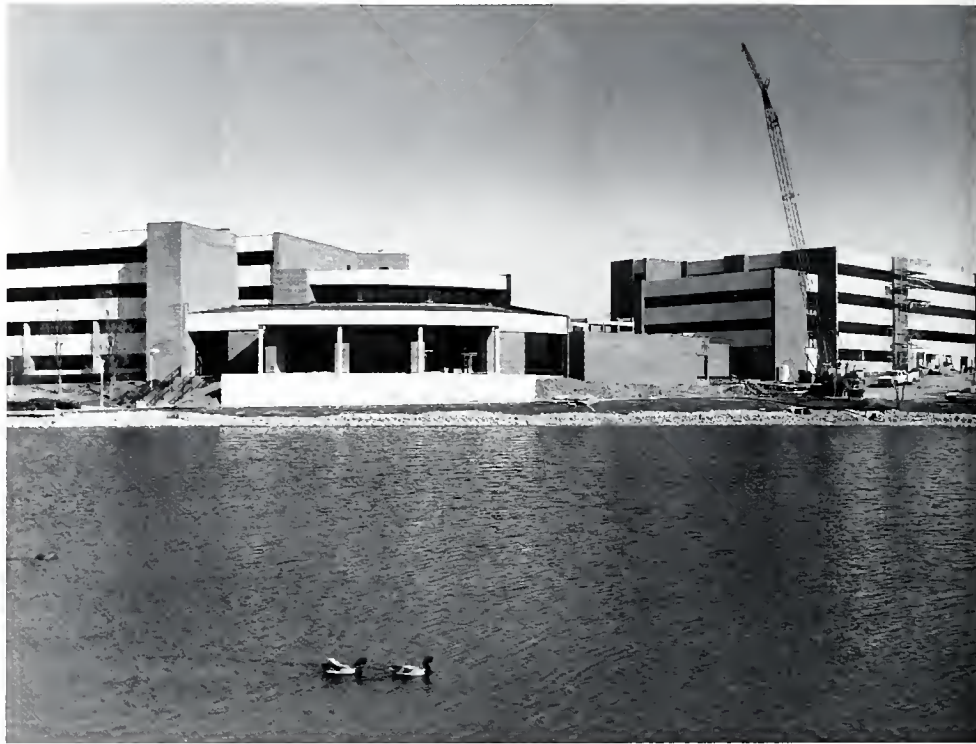
The construction of a new building is underway which will house the offices and classrooms of the Kentucky Department of Criminal Justice Training.
