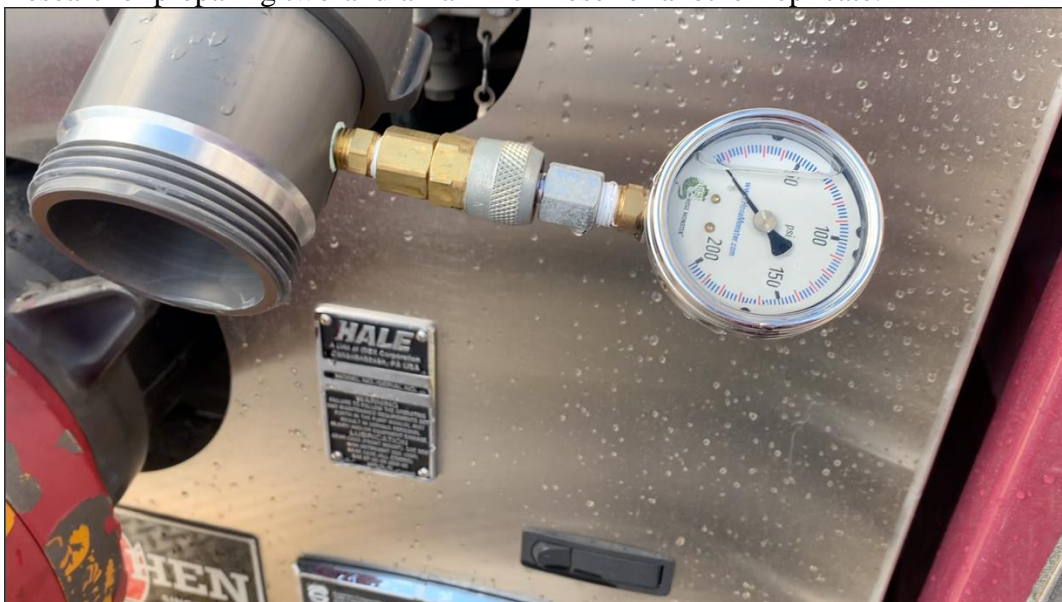
In-Line Pitot Gage used to measure pressure to determine flow.
